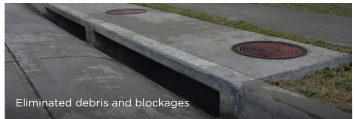
Debris and blockages
