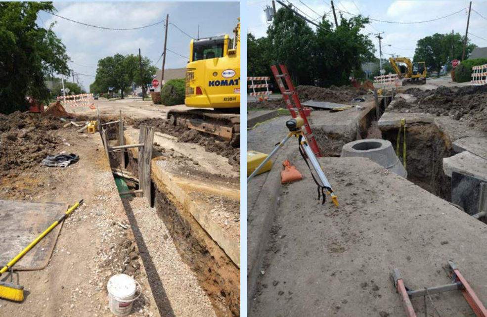
RUTH YOUNG PARK SEWER LINE
