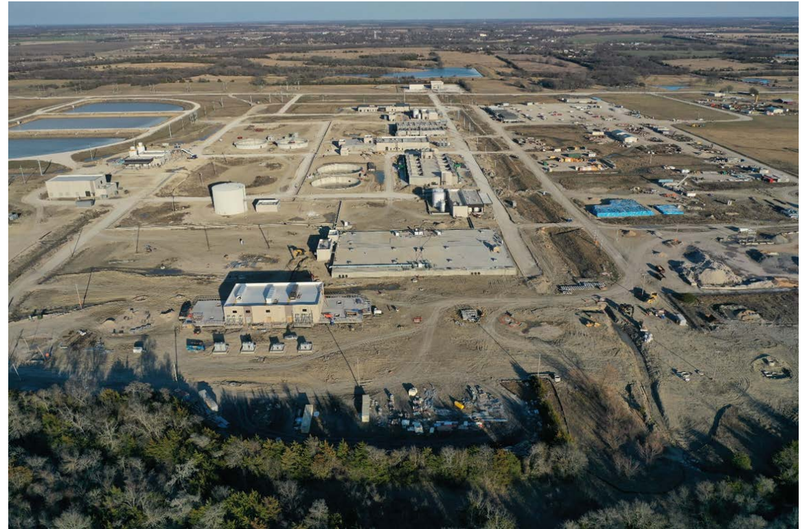
Leonard Water Treatment Plant
