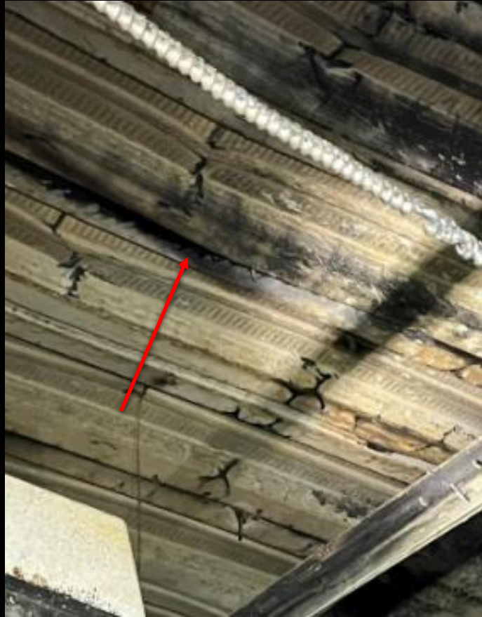
Structural Damage – Composite Deck
