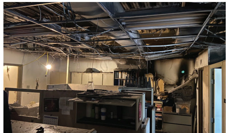
Photo taken Aug. 22, 2022 prior to any remediation.
