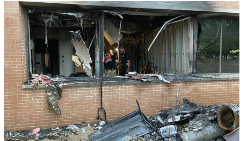
Photo taken Aug. 22, 2022 prior to any remediation.
