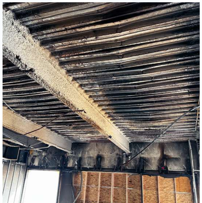
Photos taken Feb. 28, 2023 after remediation showing damage to a column (top left), electrical and communication infrastructure (top right) and the second floor slab (bottom).
