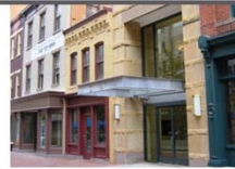
+ CANOPY STRUCTURE AND MATERIALS Cantilevered from a heavy stone base, this canopy provides a simple and strong solution to inclement weather for this entry.
