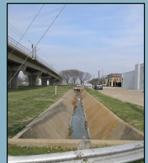
Existing drainage channel south of Belt Line Rd./Main St., east of DART rail line
